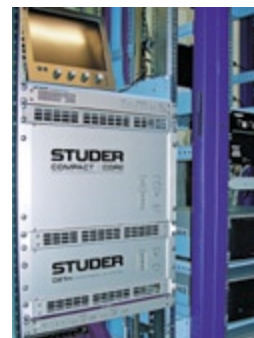
Floor specific equipment room with SCore
