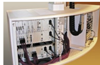
SCore installed in studio
